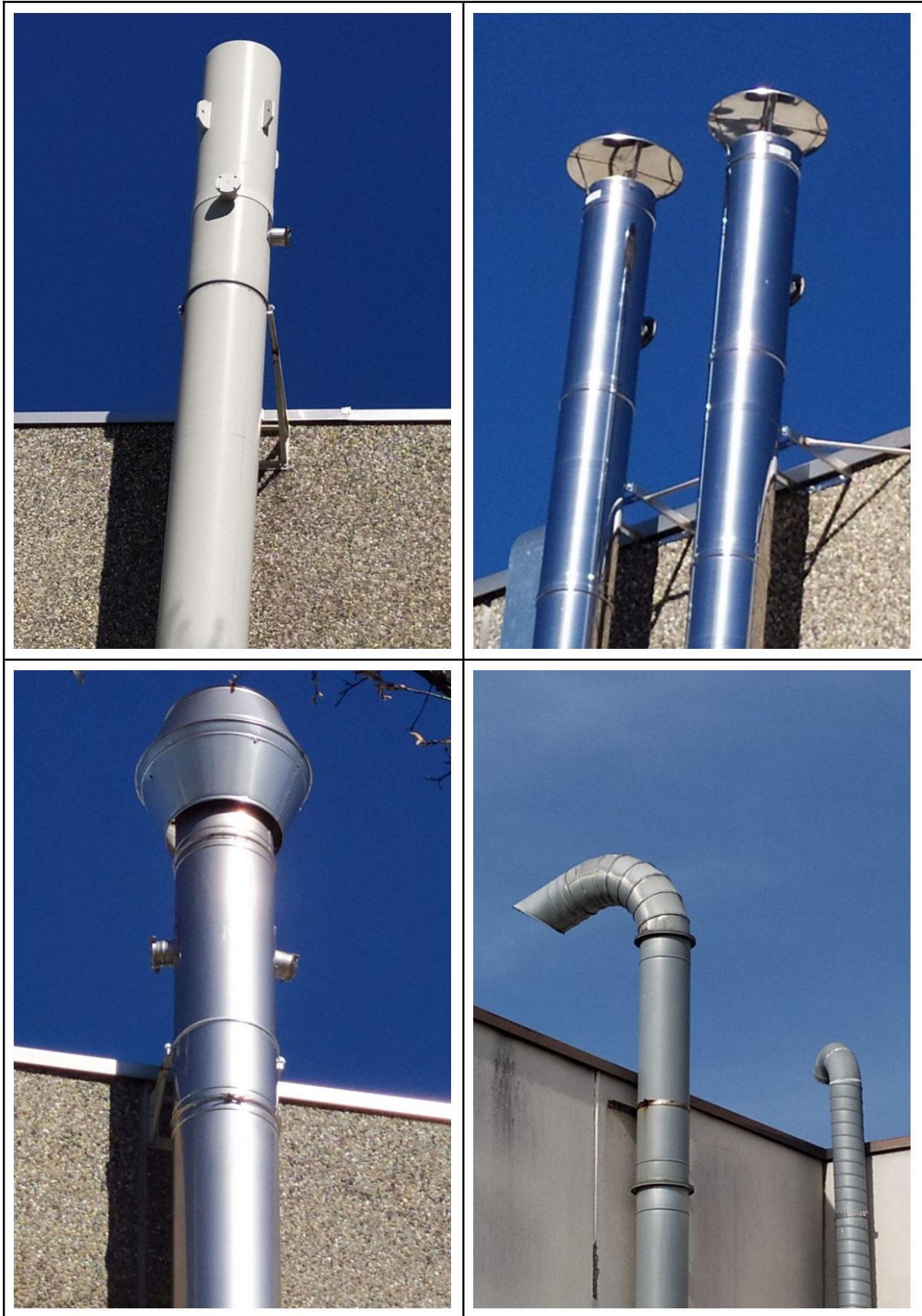
2642 Figure 4-1 Examples of point sources. Vertical stack with free discharge (top left); vertical 2643 stack with rain-cap (top right); Y-shaped vertical stack with internal rain cap (bottom left); 2644 Horizontal stack (Bottom right). (Courtesy of Enviroware)
